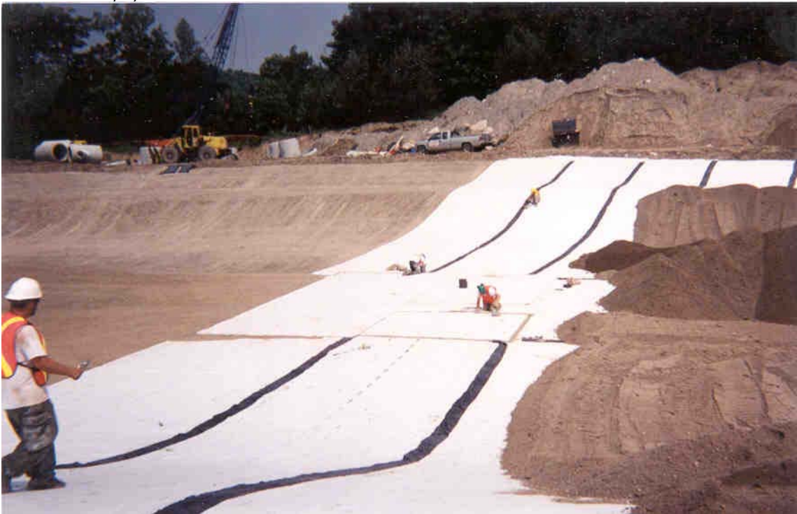
Geosynthetic Clay Liner, Bentofix, being installed by Terrafix Environmental Inc. during the summer of 2001.
