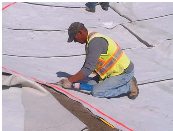
Overlaps are heat burnished with a handheld propane burner. Excess panels are cut with a utility knife (box cutters).
