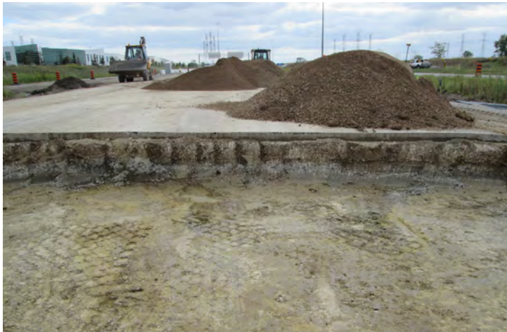
Saturated subgrade and damaged asphalt removed
