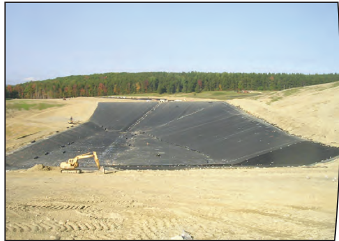
A separator geotextile is placed directly on top of the geomembrane to protect it from the 12" drainage stone layer.
