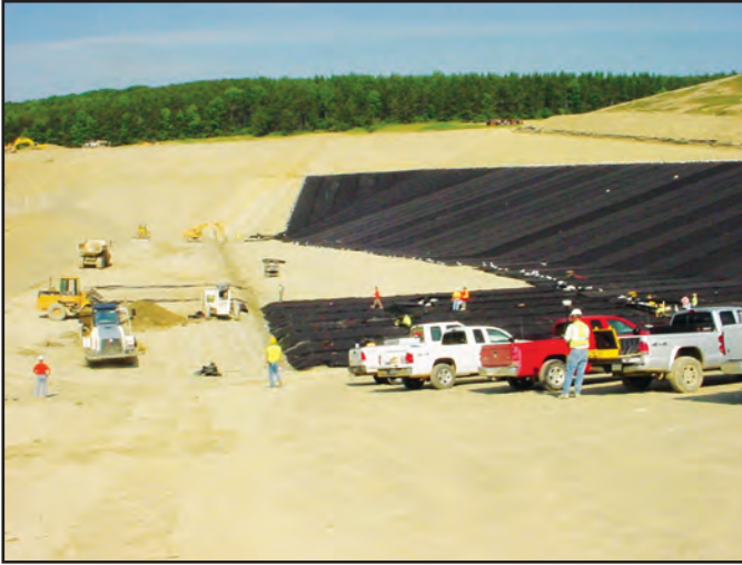
The first layer of the geocomposite for groundwater collection is deployed directly on top of the natural clay.
