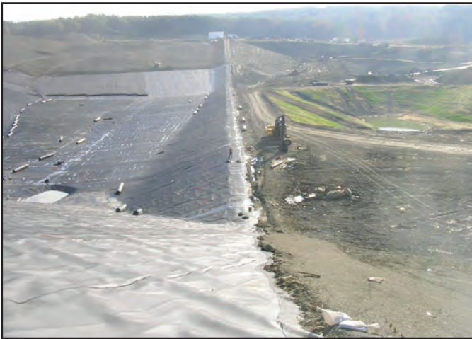
Terrafix provided a self-contained and dedicated crew to deploy, weld and test the 60 mil textured HDPE geomembrane.
