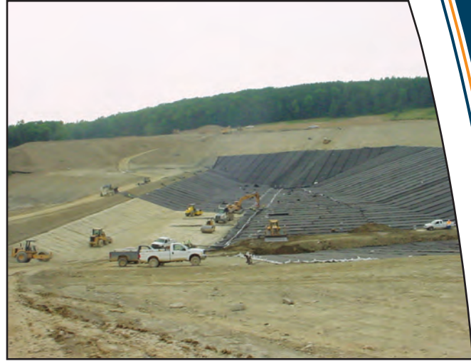
Once the secondary collection geocomposite is installed by Terrafix, the contractor begins to add the structural fill
