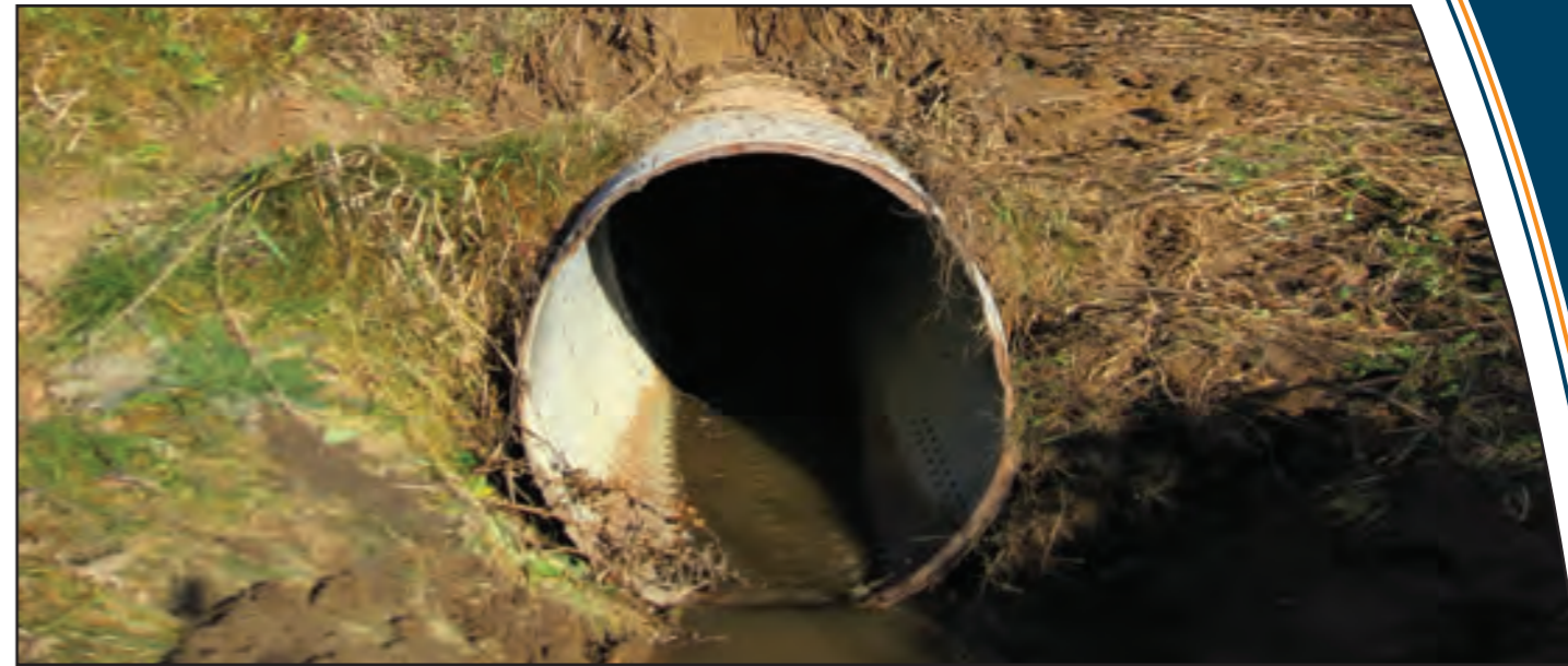
Corroded host CSP pipe.
