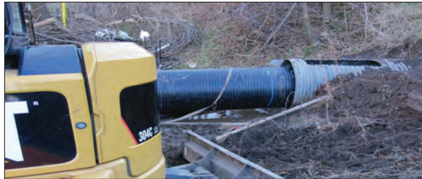
Insertion of Weholite pipe into host pipe with cut-out at top of host pipe to allow insertion of grout tube.
