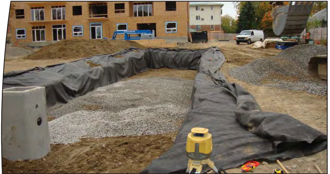
Non-woven fabric at sides of trench and 150mm of clean crushed stone for bedding
