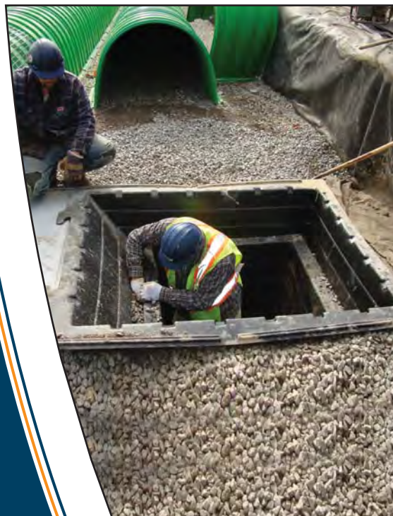
Installing bin and dumpster to adjacent floor at end of header row
