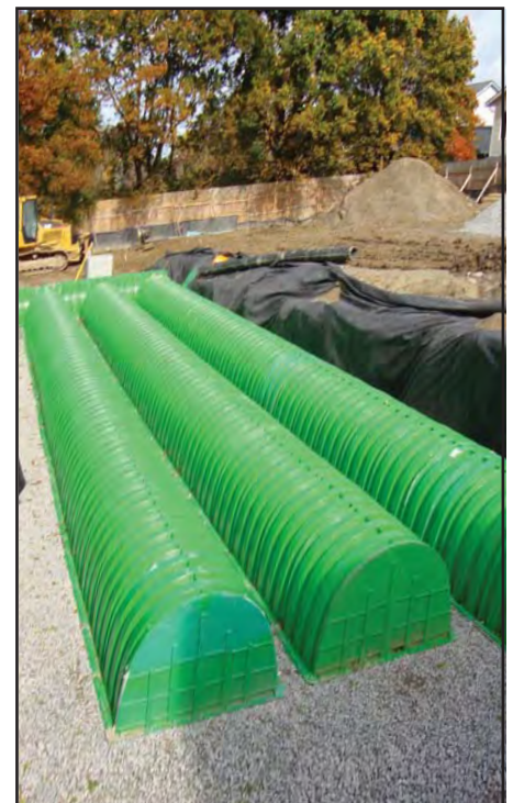
Layout of distribution rows (foreground) and header row (background)
