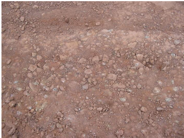
Figure 3. Subgrade full of rocks, stones, and gravel – an acceptable subgrade for a scrim-nonwoven carrier backed GCL but not for a woven only carrier GCL.
